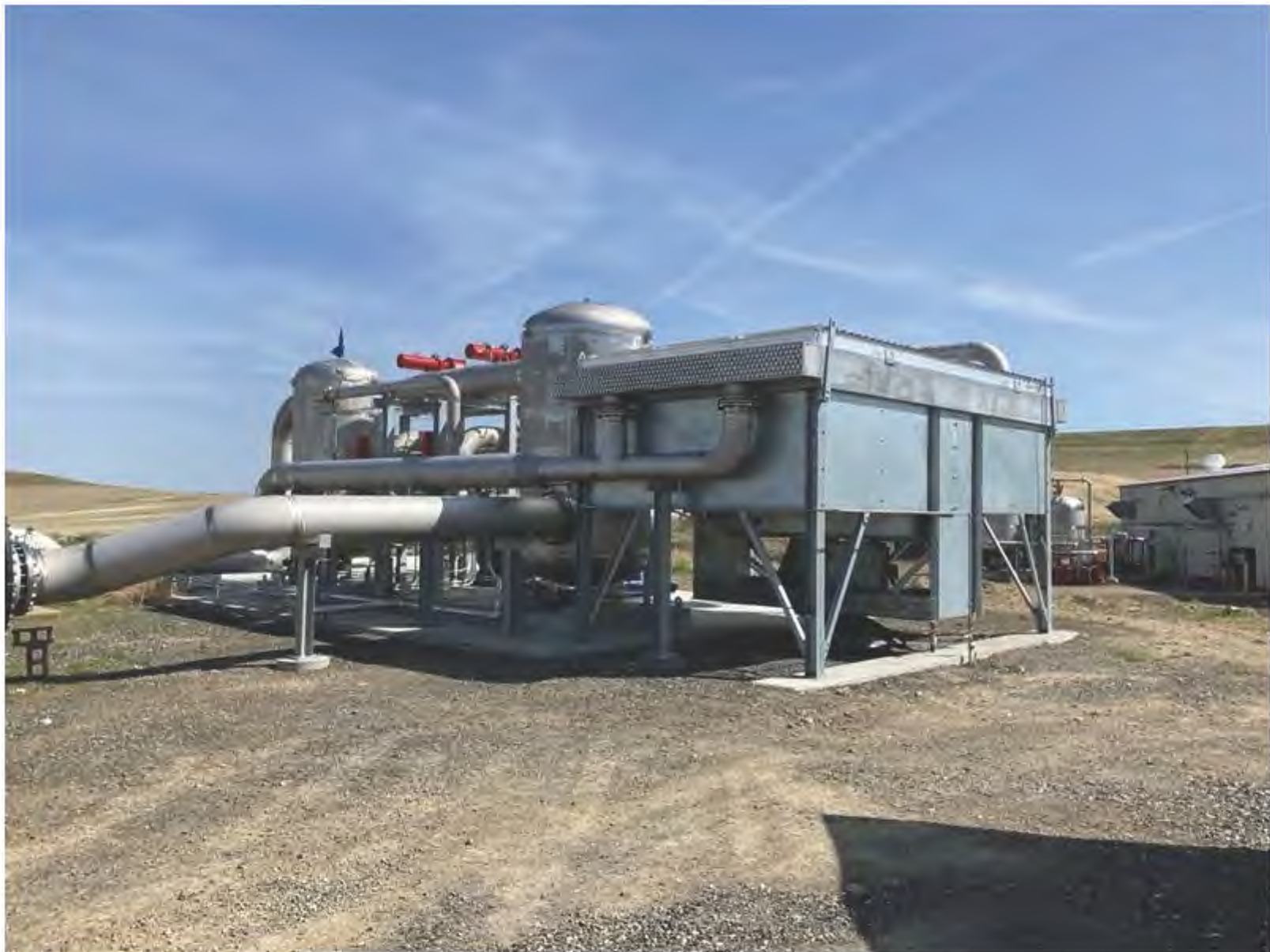
A compressor station, which is part of a landfill gas collection system
